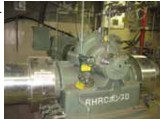
Restored cooling system pump
