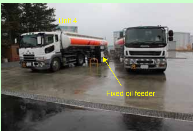
Feeding oil to the gas oil tank on the hill (underground) [Photo taken on March 27, 2013]
