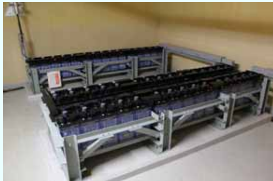
After function check (battery) [Permanent installation completed on March 14, 2013] (Photo taken on March 14, 2013)
