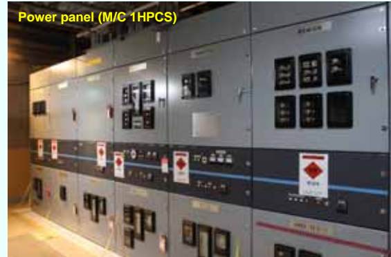
After function check [Permanent installation completed on March 1, 2013] (Photo taken on March 12, 2013)
