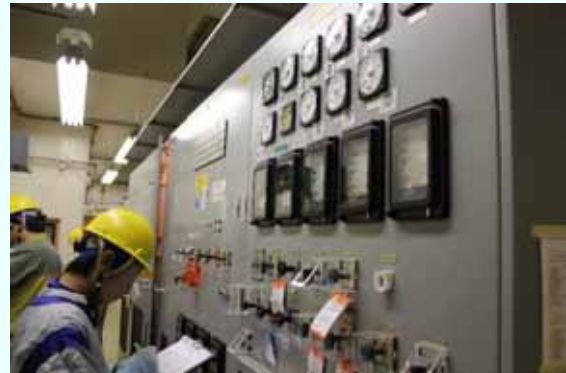
Trial operation (control panel) [Permanent installation completed on March 21, 2013] (Photo taken on March 19, 2013)
