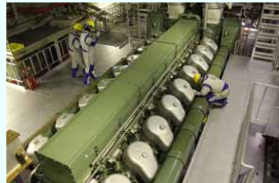
Trial operation (upper part of the diesel engine) [Permanent installation completed on March 21, 2013] (Photo taken on March 21, 2013)
