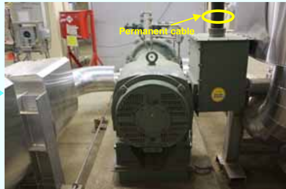
Switching to the permanent cable completed for the electric motor of the emergency diesel generator cooling system (B) [Permanent installation completed on March 1, 2013] (Photo taken on April 1, 2013)
