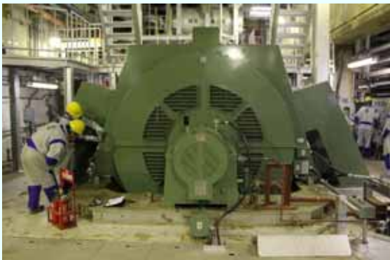
Trial operation (generator) [Permanent installation completed on March 21, 2013] (Photo taken on March 21, 2013)
