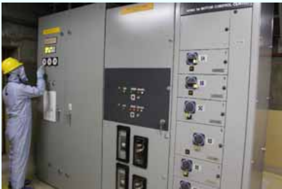
After function check (charger panel) [Permanent installation completed on March 12, 2013] (Photo taken on April 1, 2013)
