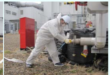
Connecting the fire hose (Unit 2)
