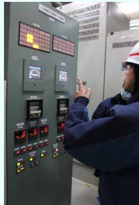
Function check [Permanent installation completed on February 18, 2013] (Photo taken on February 12, 2013)
