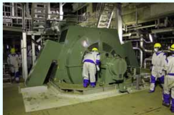
Trial operation (generator) [Permanent installation completed on February 13, 2013] (Photo taken on February 1, 2013)
