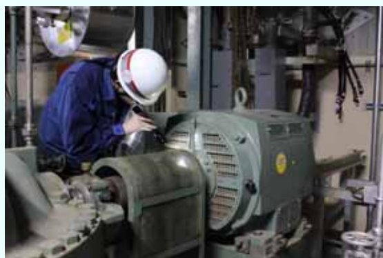
Trial operation of the electric motor of the residual heat removal system cooling system pump (A) [Permanent installation (A&C) completed on February 12, 2013] (Photo taken on February 7, 2013)
