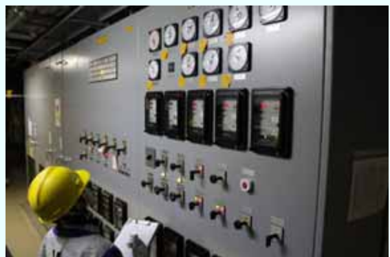
Trial operation (control panel) [Permanent installation completed on February 13, 2013] (Photo taken on February 1, 2013)
