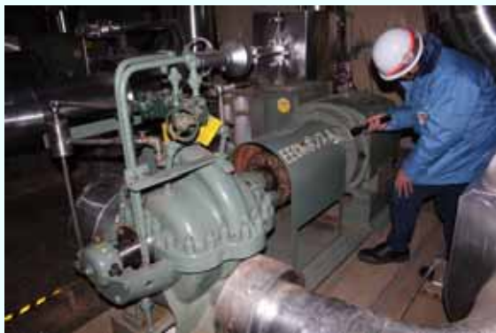
Trial operation of the electric motor of the emergency diesel generator cooling system (A) [Permanent installation completed on February 5, 2013] (Photo taken on February 5, 2013)
