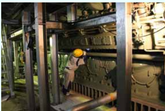
Trial operation (lower part of the diesel engine) [Permanent installation completed on February 1, 2013] (Photo taken on February 1, 2013)
