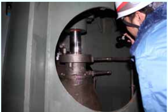
Trial operation of the electric motor of the residual heat removal system cooling seawater system pump (C) [Permanent installation completed on February 8, 2013] (Photo taken on February 8, 2013)
