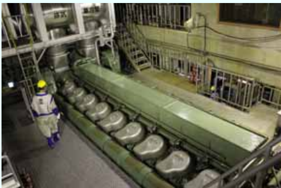
Trial operation (upper part of the diesel engine) [Permanent installation completed on February 1, 2013] (Photo taken on February 1, 2013)
