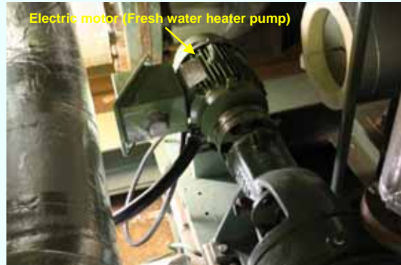
Electric motor (Fresh water heater pump* 1 ) installation completed (Photo taken on February 27, 2013)
