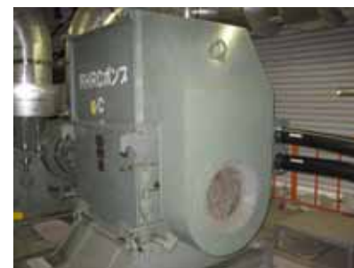
Restored cooling system pump
