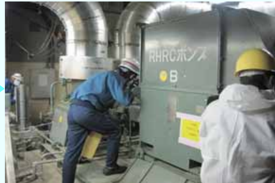
Trial operation of the electric motor of the residual heat removal system cooling system pump (B) [Permanent installation completed on January 28, 2013] (Photo taken on January 28, 2013)
