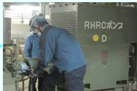
Trial operation of the electric motor of the residual heat removal system cooling system pump (D) [Permanent installation completed on January 28, 2013] (Photo taken on January 28, 2013)
