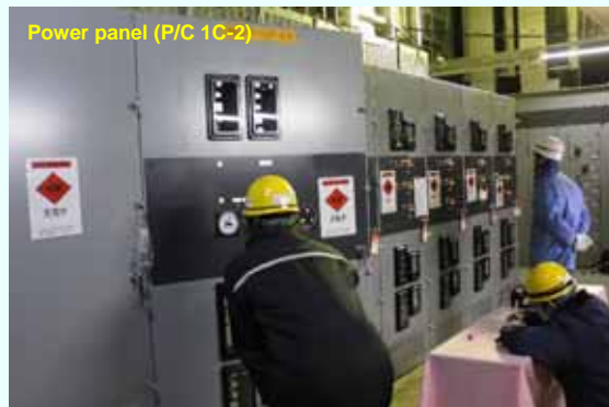
Function check [Permanent installation completed on January 28, 2013] (Photo taken on January 28, 2013)
