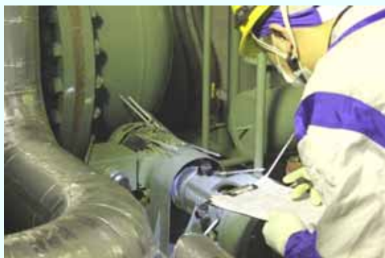
Trial operation of the electric motor (Fresh water heater pump*1) (Photo taken on January 24, 2013)
