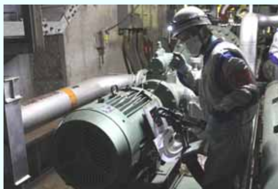
Trial operation of the electric motor (Lubricating oil priming pump*2) [Permanent installation completed on January 31, 2013] (Photo taken on January 24, 2013)
