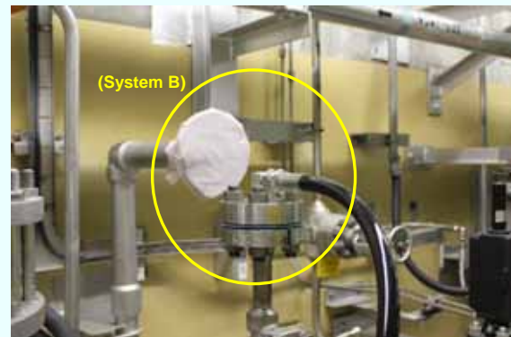
Temporary hose connection for system B (Enlarged image) (December 14, 2012)
