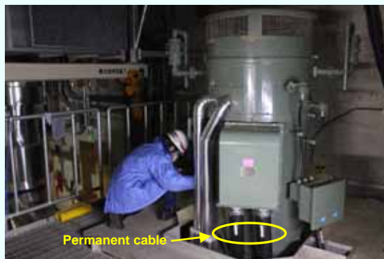
Trial operation of the electric motor of the residual heat removal system cooling seawater system pump (D) [Permanent installation completed on January 30, 2013] (Photo taken on January 30, 2013)
