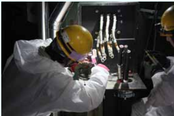
Taking cable core out of the permanent cable for the electric motor of the residual heat removal system cooling seawater system pump (D) (Photo taken on January 22, 2013)
