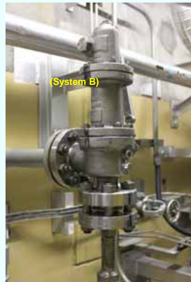
Permanent pipe (valve) connection for system B (Enlarged image) (Photo taken on January 24, 2013)
