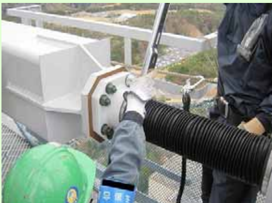
Seismic control oil damper installation (Photo taken on April 20, 2012)
