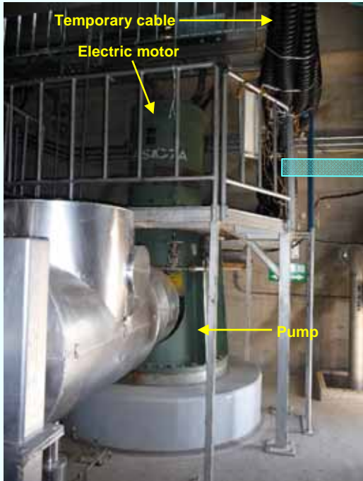
Full view of the residual heat removal equipment cooling seawater system pump (A) (Photo taken on September 13, 2012)
