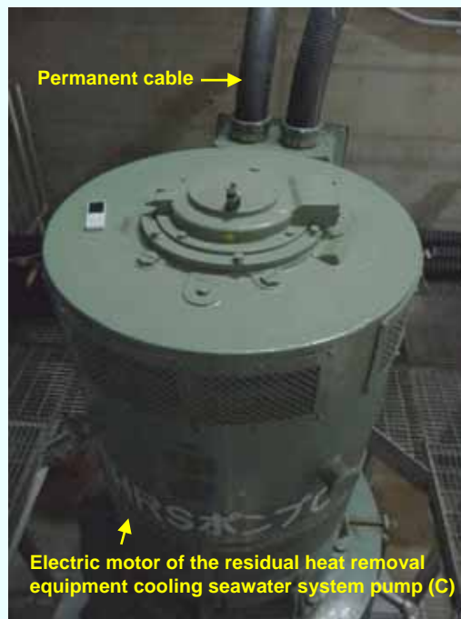
Permanent cable installation for the electric motor of the residual heat removal equipment cooling seawater system pump (C) (Permanent installation completed on September 11, 2012) (Photo taken on September 13, 2012)
