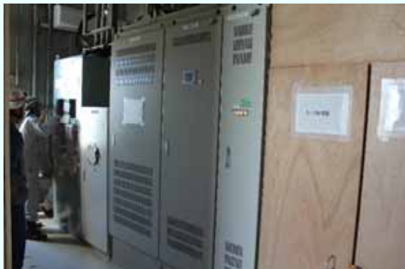
Control board installation (Photo taken on September 4, 2012)
