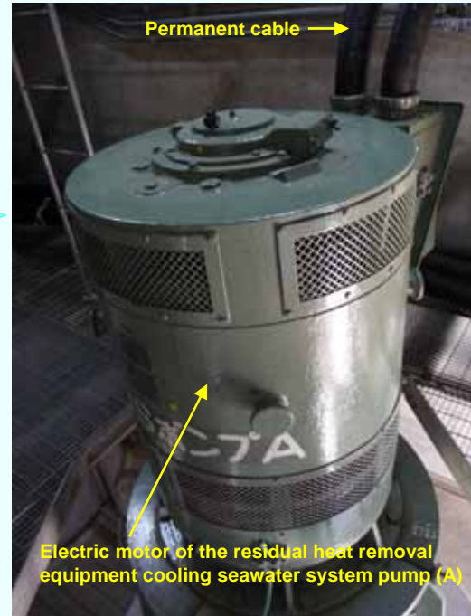
Permanent cable installation for the electric motor of the residual heat removal equipment cooling seawater system pump (A) (Permanent installation completed on September 11, 2012) (Photo taken on September 13, 2012)
