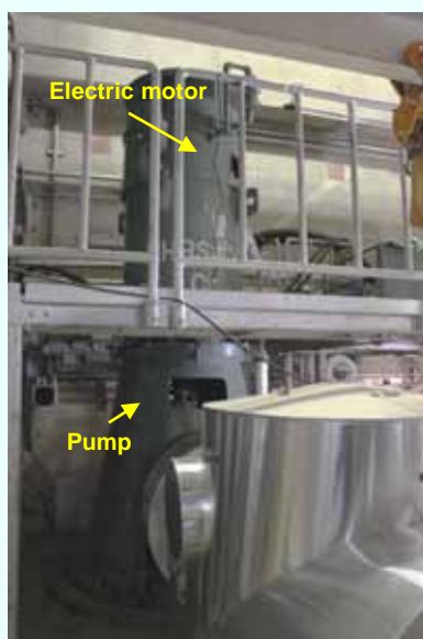
Full view of the residual heat removal equipment cooling seawater system pump (C) (Photo taken on September 26, 2012)
