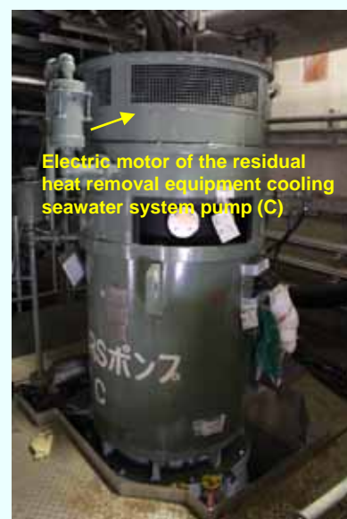
Installation of the electric motor of the residual heat removal equipment cooling seawater system pump (C) (Completed on September 13, 2012) (Photo taken on September 26, 2012)
