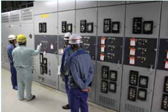
Functional check of power panel (P/C 3C-2) (Permanent installation completed on August 27, 2012) (Photo taken on August 27, 2012)
