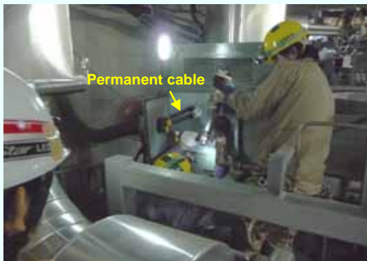
Switching to the permanent cable for the electric motor of the residual heat removal equipment cooling system pump (C) (Photo taken on September 13, 2012)
