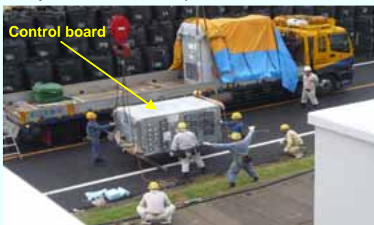
Control board being lifted up by a crane truck (Photo taken on September 21, 2012)
