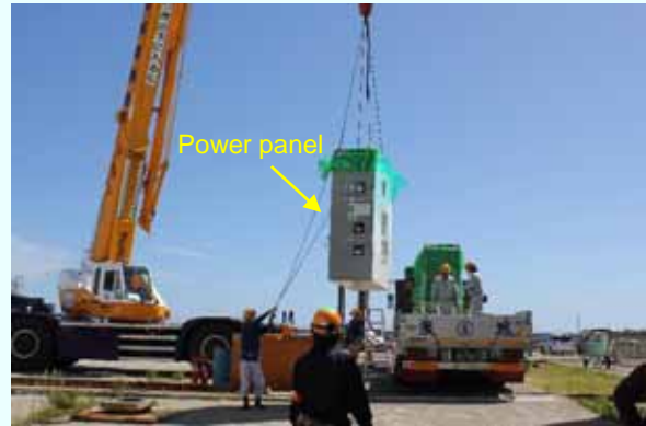
1. Power panel being lifted up by a crane truck (Photo taken on September 3, 2012)
