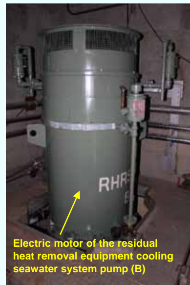
Installation of the electric motor of the residual heat removal equipment cooling seawater system pump (B) (Completed on September 11, 2012) (Photo taken on September 26, 2012)
