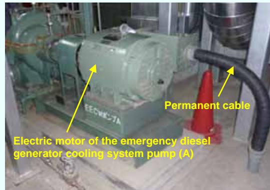
Permanent cable installation for the electric motor of the emergency diesel generator cooling system pump (A) (Permanent installation completed on September 6, 2012) (Photo taken on September 13, 2012)
