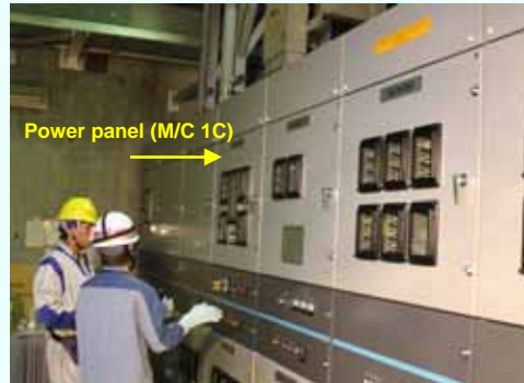
Functional check (Completed on September 27, 2012) (Photo taken on September 27, 2012)
