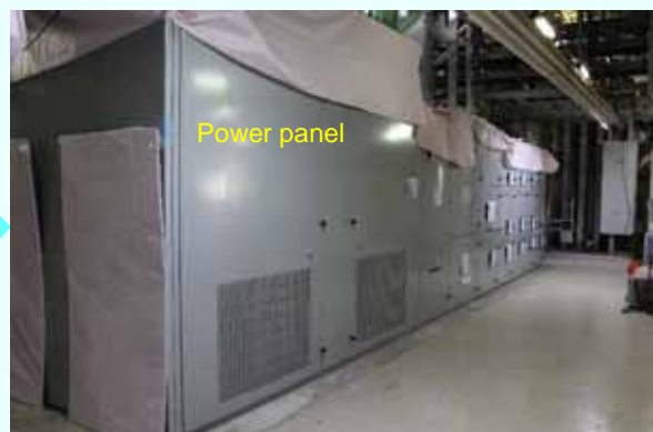
5. Power panel (P/C 2C-2) installation (Completed on September 11, 2012) (Photo taken on September 26, 2012)
