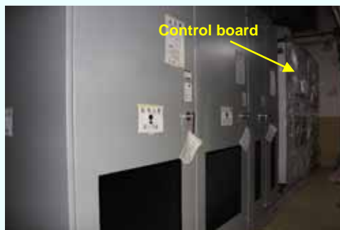
Carry-in of the control board etc. into the building (Completed on September 21, 2012) (Photo taken on September 26, 2012)
