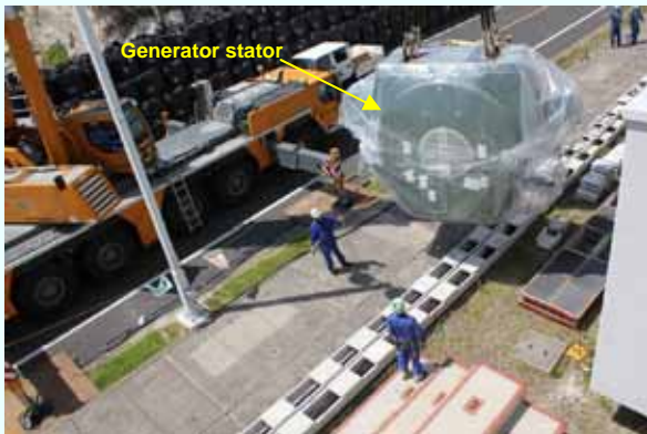
1. Generator stator being lifted up by a crane car (Photo taken on August 7, 2012)
