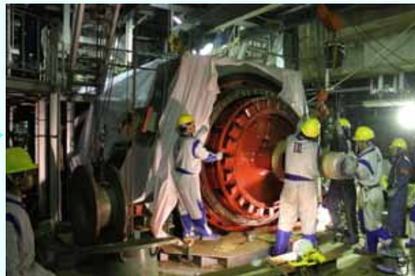
8. Generator rotor being inserted into the generator stator (Photo taken on August 22, 2012)
