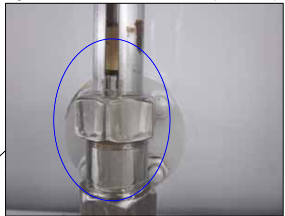
Leaking section at the center connection (NO.4 tank)
