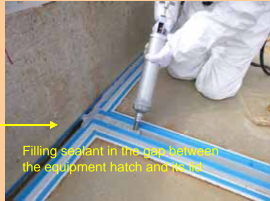
Filling sealant in the gap between the equipment hatch and its lid (Photo taken on March 23, 2012)
