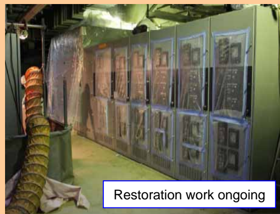
Unit 1 power panel (P/C 1D-2) on the 1st floor of Unit 1 Seawater Heat Exchanger Building Currently in the process of installing the newly manufactured power panel (Photo taken on June 18, 2012)
