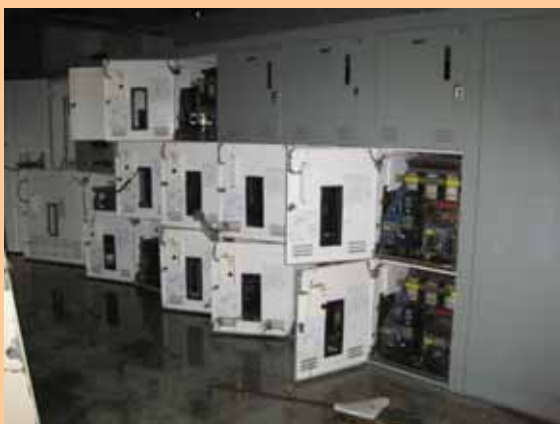
Unit 1 power panel (P/C 1D-2) on the 1st floor of Unit 1 Seawater Heat Exchanger Building (Photo taken on March 13, 2011)
