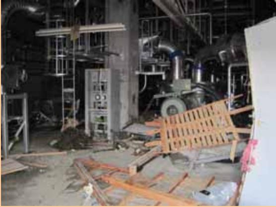
Unit 4 residual heat removal system cooling (C system) on the 1st floor of Unit 4 Seawater Heat Exchanger Building (Photo taken on March 13, 2011)
