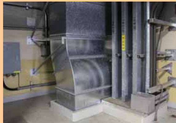
Air conditioning duct on the 1st floor of Unit 1 Seawater Heat Exchanger Building Restoration completed with the damaged parts replaced/repaired (Photo taken on June 18, 2012)
