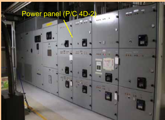
Power panel (P/C 4D-2) (Photo taken on June 18, 2012)
