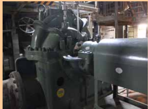
Reactor component cooling system pump (B) on the basement of Unit 4 Seawater Heat Exchanger Building Restoration completed (Cleaning and inspection were done) (Photo taken on June 18, 2012)
