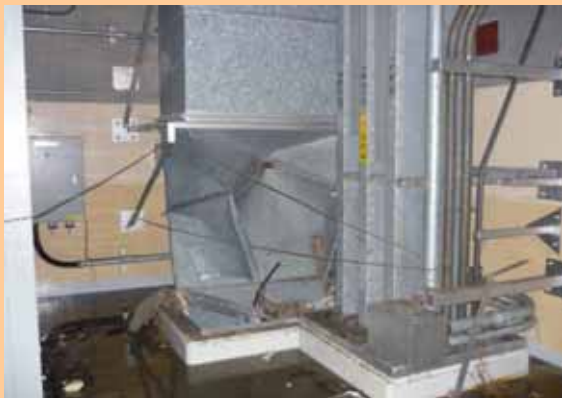
Air conditioning duct on the 1st floor of Unit 1 Seawater Heat Exchanger Building (Photo taken on March 16, 2011)
