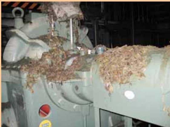
Reactor component cooling system pump (B) on the basement of Unit 4 Seawater Heat Exchanger Building (Photo taken on March 23, 2011)
