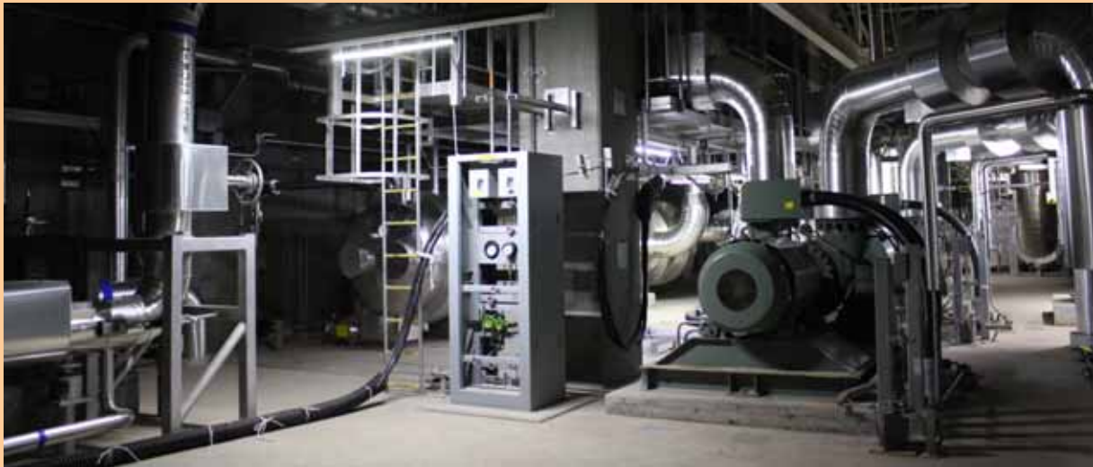
Unit 4 Seawater Heat Exchanger Building 1st Floor after restoration (Photo taken on June 30, 2012)
