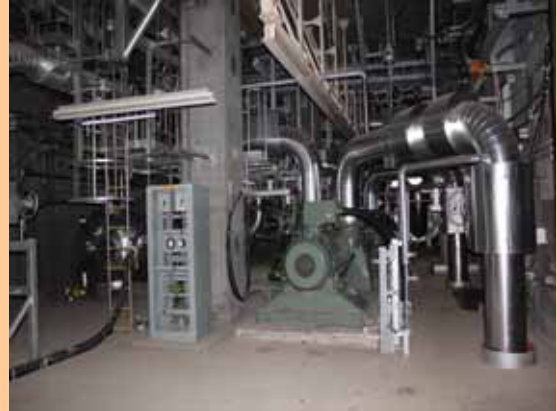
Unit 4 residual heat removal system cooling (C system) on the 1st floor of Unit 4 Seawater Heat Exchanger Building Electric motor repair and floor cleaning have been completed (Photo taken on June 7, 2012)
