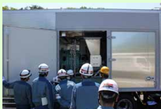
Training: Air-cooled gas turbine power supply car (Photo taken on June 27, 2012)
