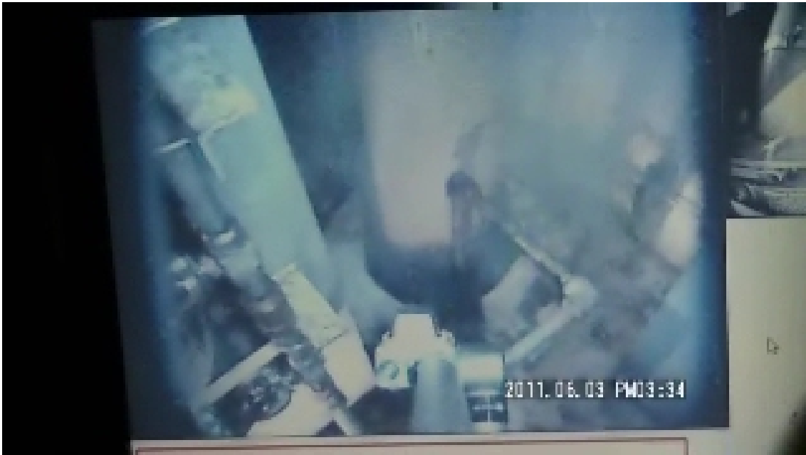
Attached Figure 2. Steam Released from Floor Penetration on Unit 1 R/B First Floor (Photo taken on June 3, 2011)
