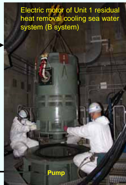
2. Installation of the electric motor of Unit 1 residual heat removal cooling sea water system (B system) (Photo taken on April 5, 2012)
