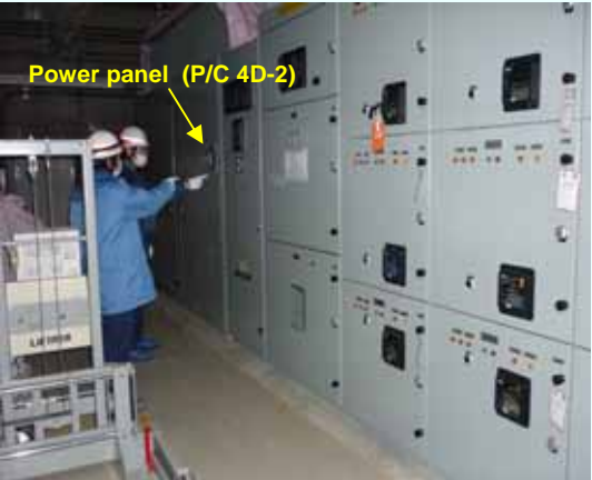
Permanent installation of power panel (P/C 4D-2) has been completed on March 23, 2012 (Photo taken on March 23, 2012)
