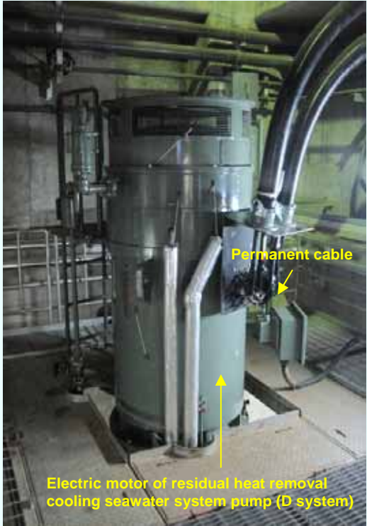
Switching to the permanent cable for the electric motor of residual heat removal cooling seawater system pump (D system) (Completed / photo taken on April 25, 2012)
