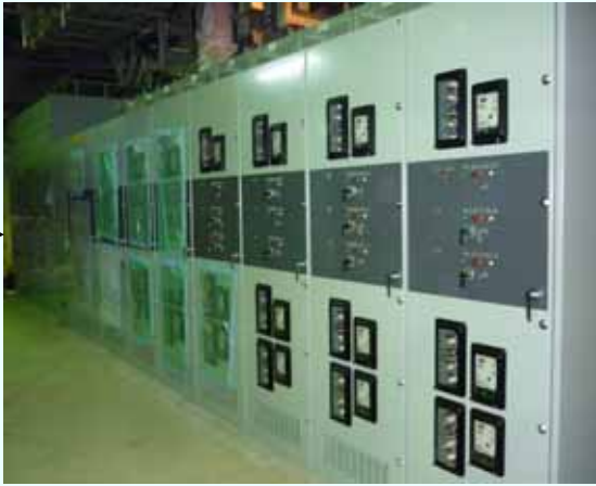
4. Power panel (P/C 1C-1) installation completed on April 19 (Photo taken on April 23, 2012)
