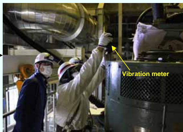
4. Function check after installation (Vibration measurement during the trial run) (Photo taken on April 12)
