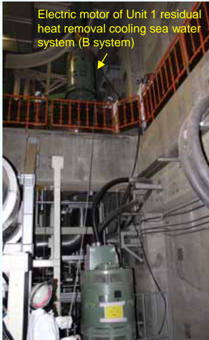
1. Moving the electric motor of Unit 1 residual heat removal cooling sea water system (B system) from the 2nd floor to the 1st floor of the Sea Water Heat Exchanger Building (Photo taken on April 5, 2012)
