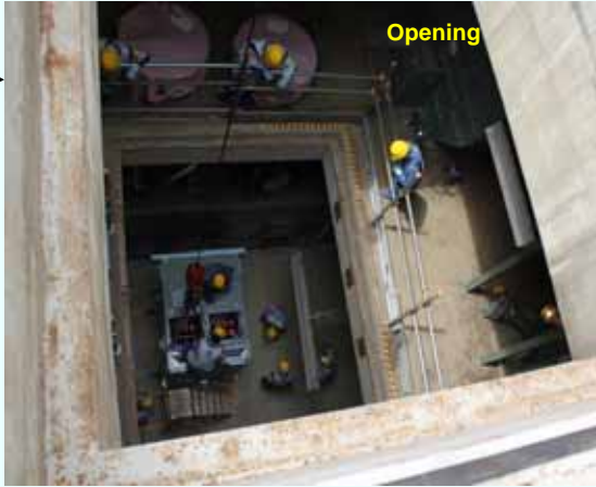
2. Power panel (P/C 1C-1) carried down through the opening (Photo taken on April 13, 2012)
