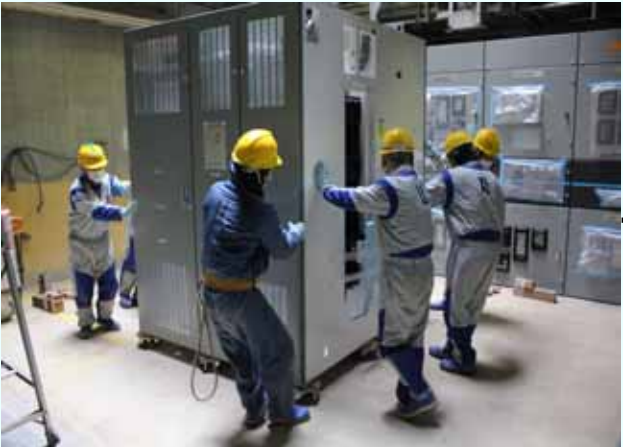
3. Moving the power panel (P/C 1C-1) after it's lifted down (Photo taken on April 13, 2012)
