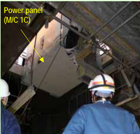
(2) Lift up and entry (Lift down to the installation location) (Photo on March 15, 2012)
