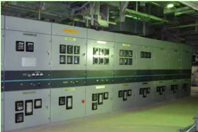
(4) Installation of the power panel (M/C 1C) was completed (Installation was completed on March 28, 2012) (Photo on April 2, 2012)
