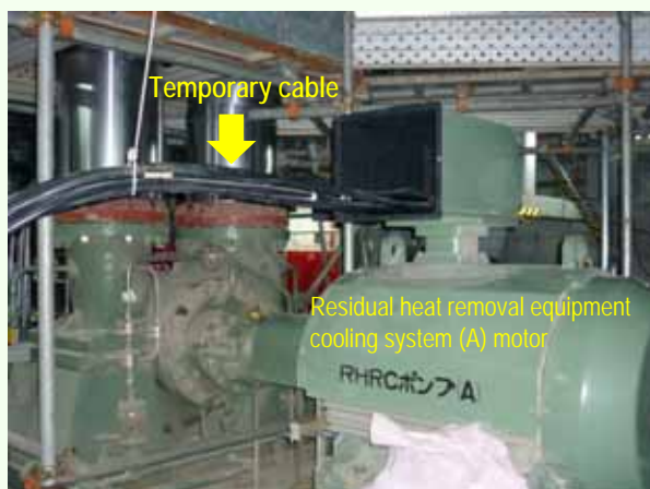
Temporary cable connection (Photo on February 24, 2012)
