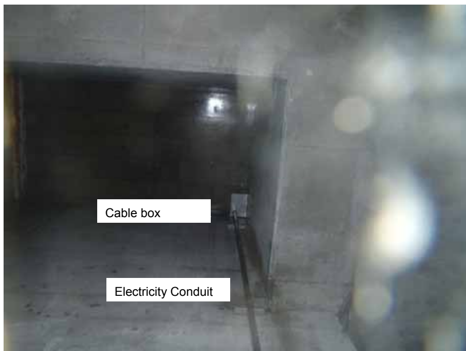
【Photo 1】 Situation of accumulated water in the trench
