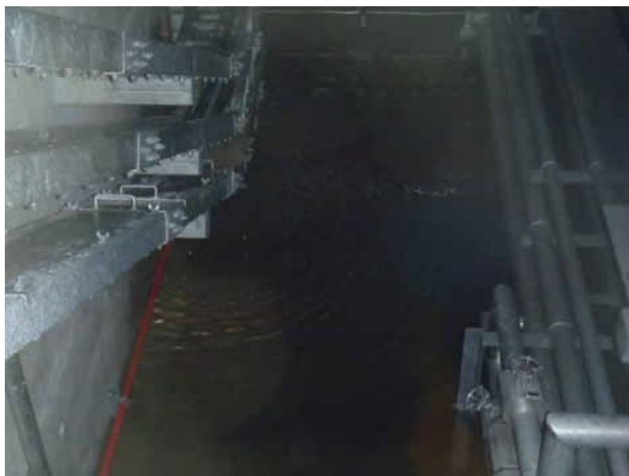
【Photo 2】 Situation of accumulated water in the trench
