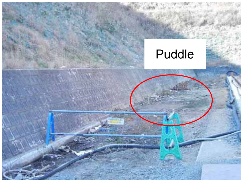
Figure3 Water incursion to cable conduit line
