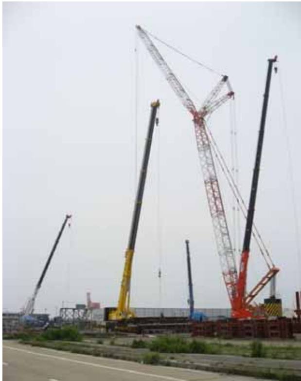
Photo 1 Tentative assembly of reactor building's cover unit by crawler crane ( Onahama port )
