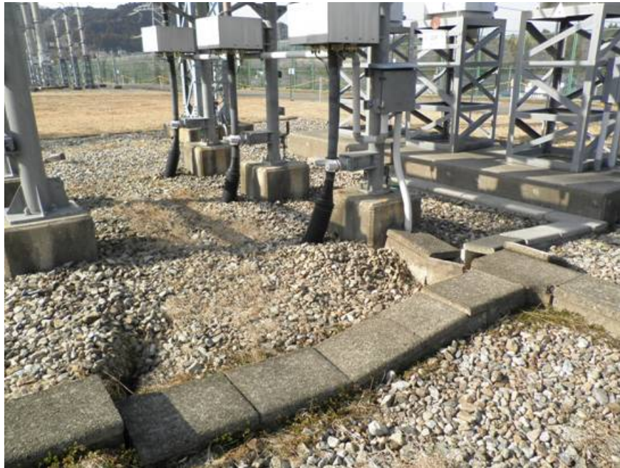
Photo : Tokyo Electric Power Company, March 12, 2011
