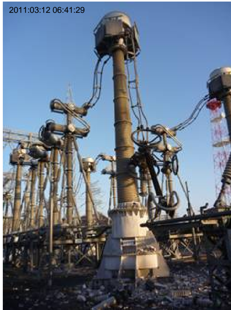
Photo : Tokyo Electric Power Company, March 12, 2011
