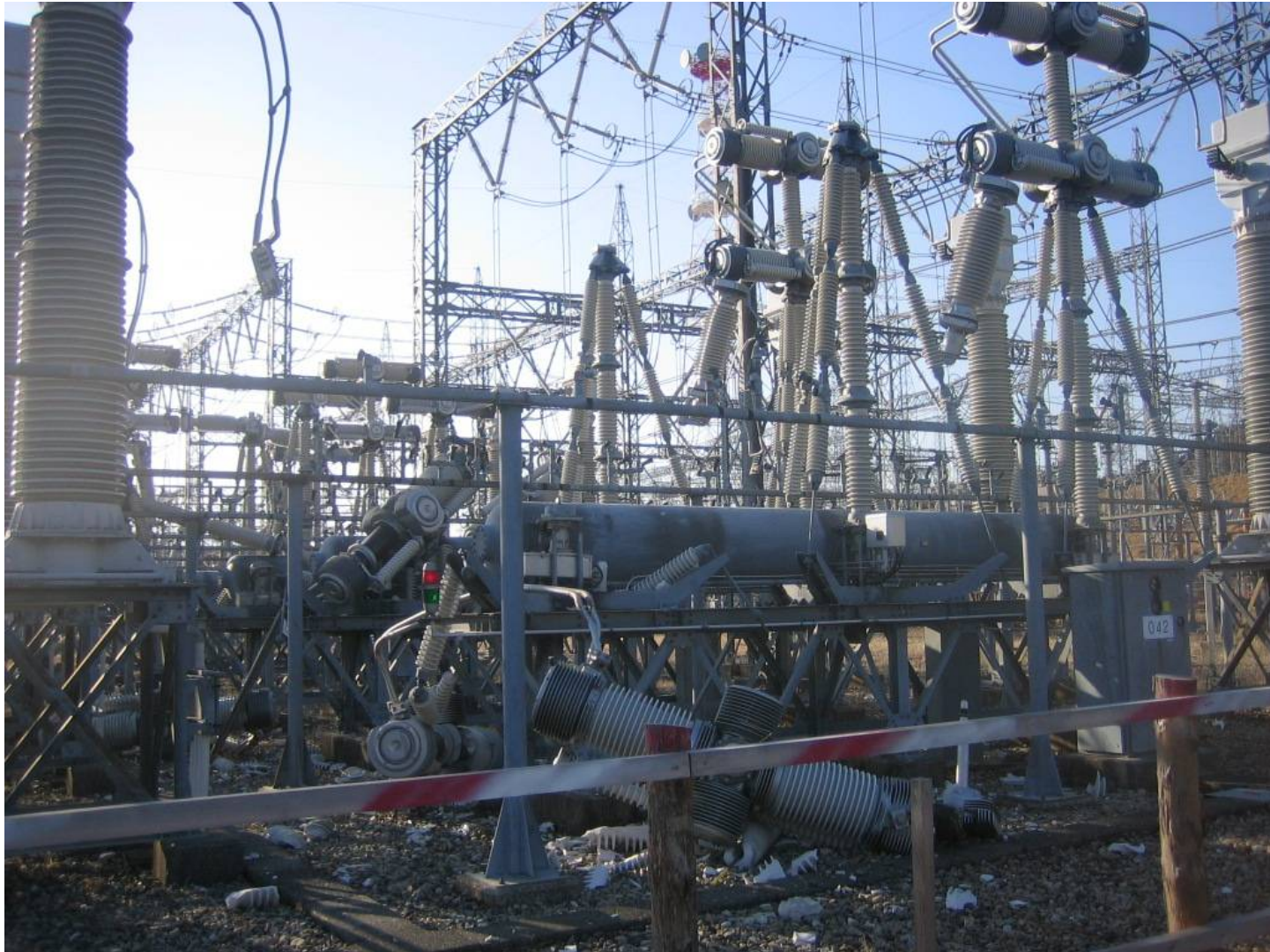
Photo : Tokyo Electric Power Company, March 11, 2011
