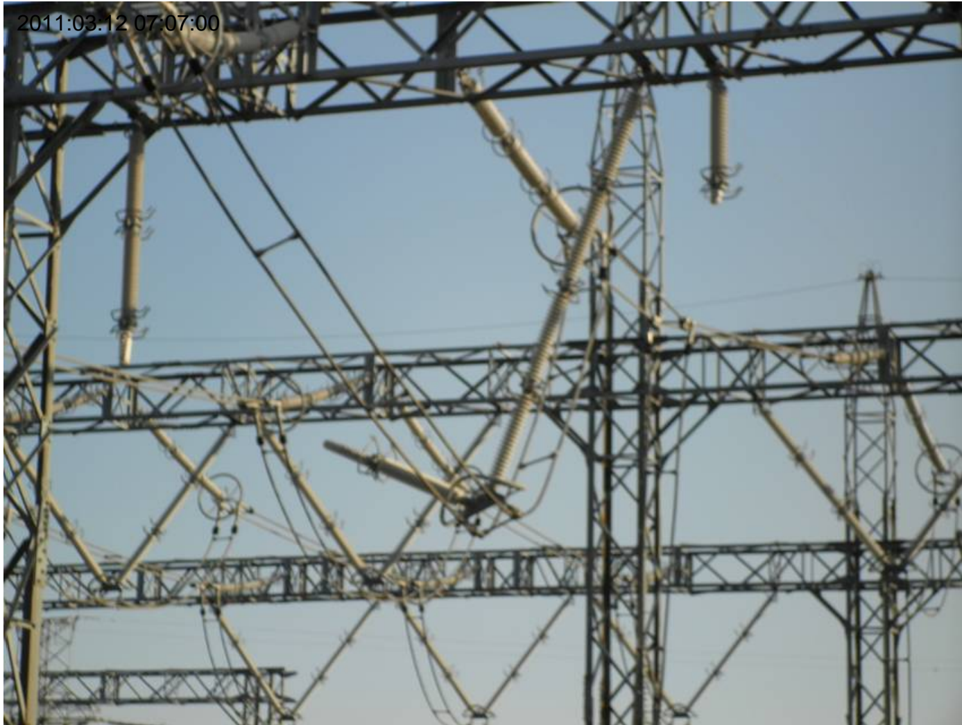
Photo : Tokyo Electric Power Company, March 12, 2011
