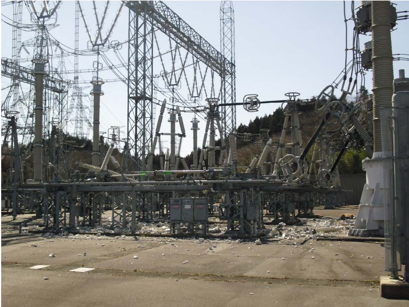
Photo : Tokyo Electric Power Company, March 11, 2011
