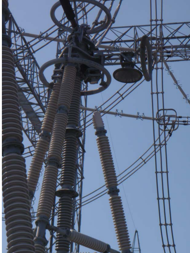
Photo : Tokyo Electric Power Company, March 12, 2011
