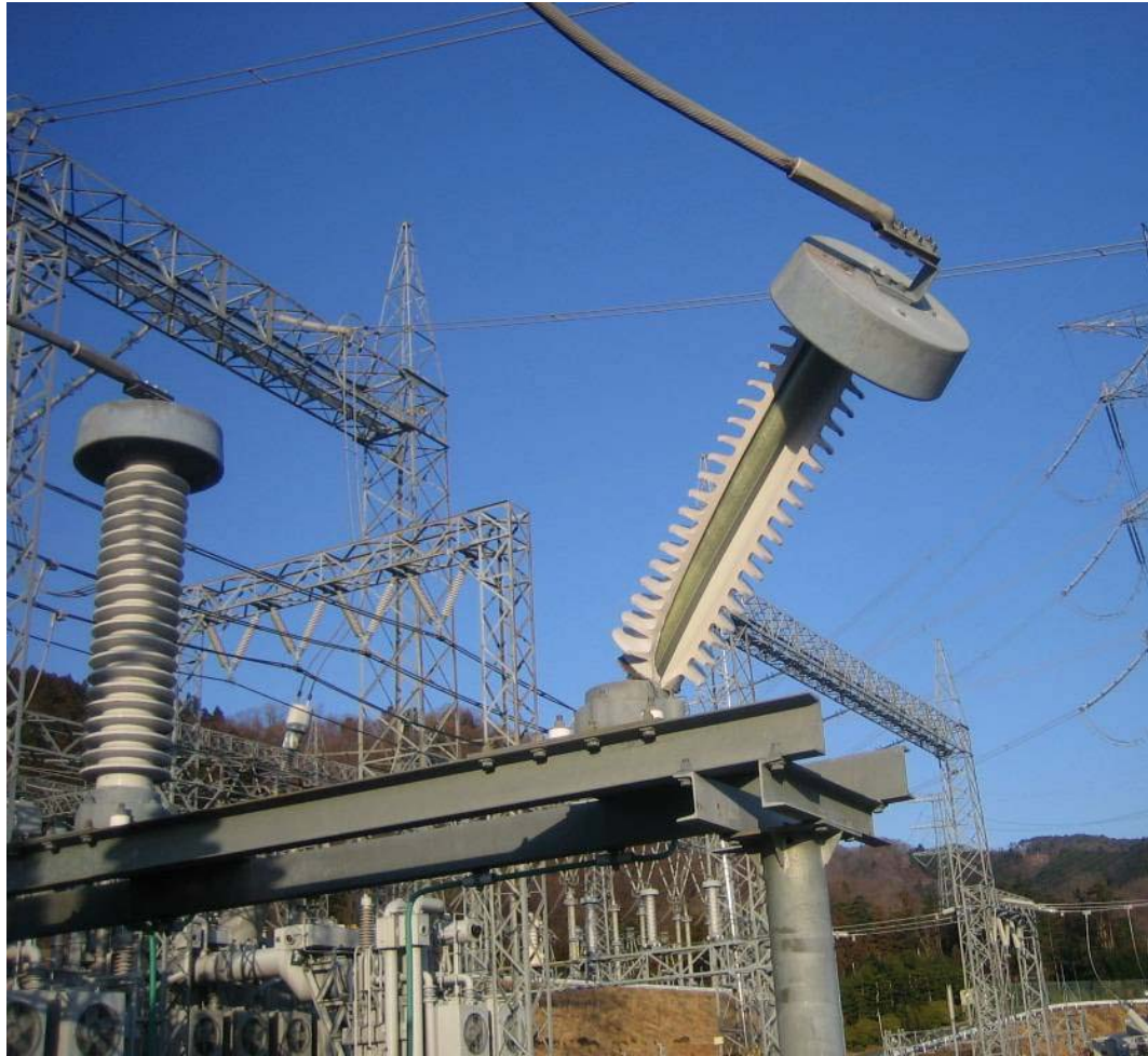
Photo : Tokyo Electric Power Company, March 12, 2011
