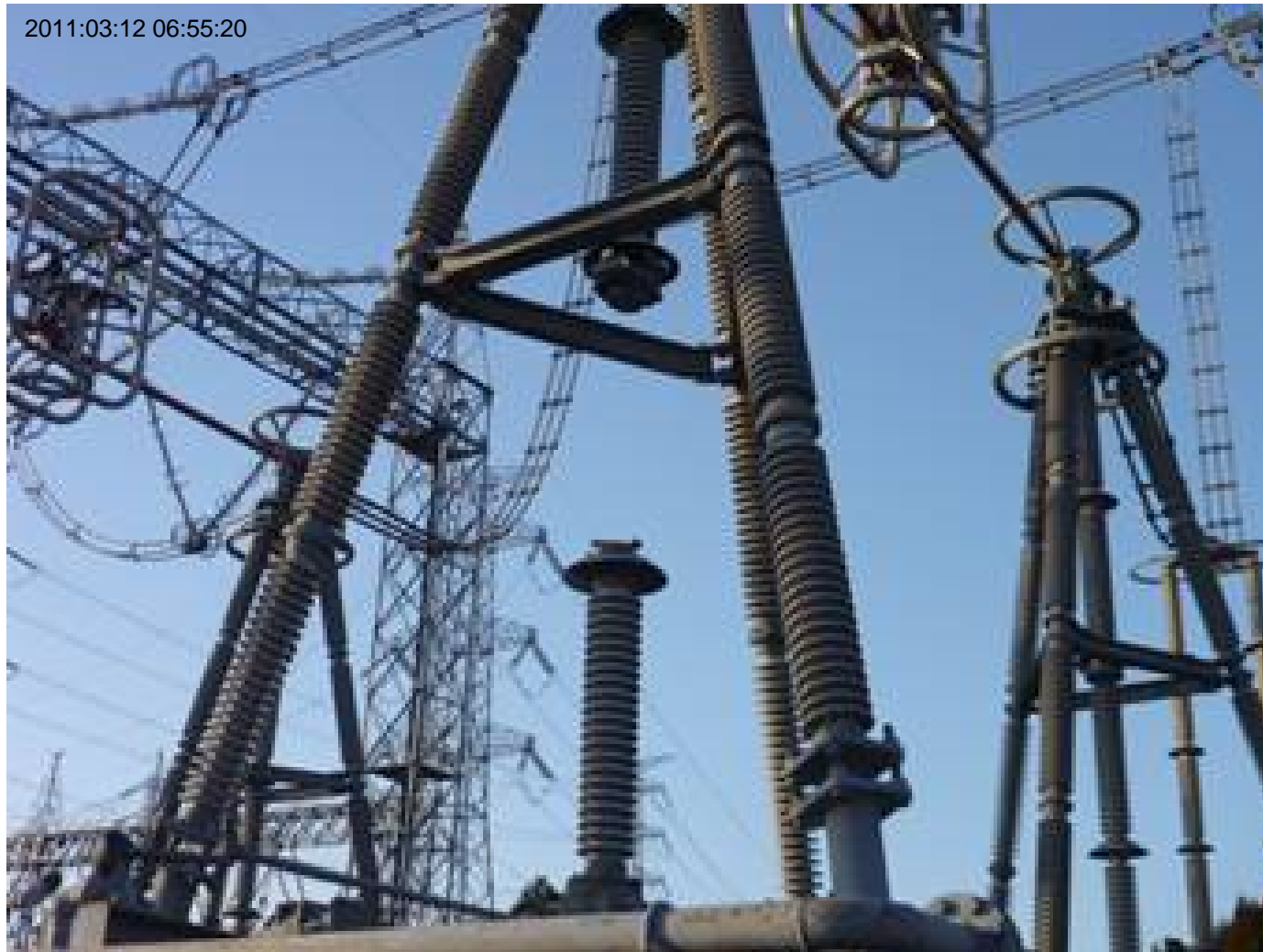
Photo : Tokyo Electric Power Company, March 12, 2011
