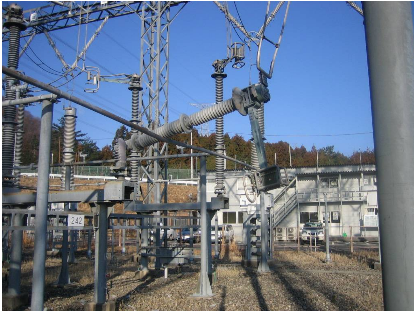
Photo : Tokyo Electric Power Company, March 12, 2011
