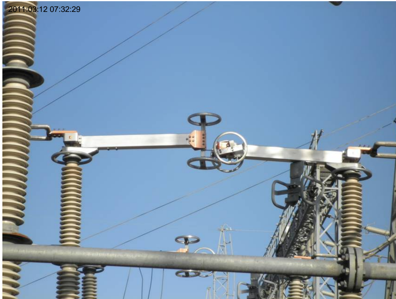
Photo : Tokyo Electric Power Company, March 12, 2011
