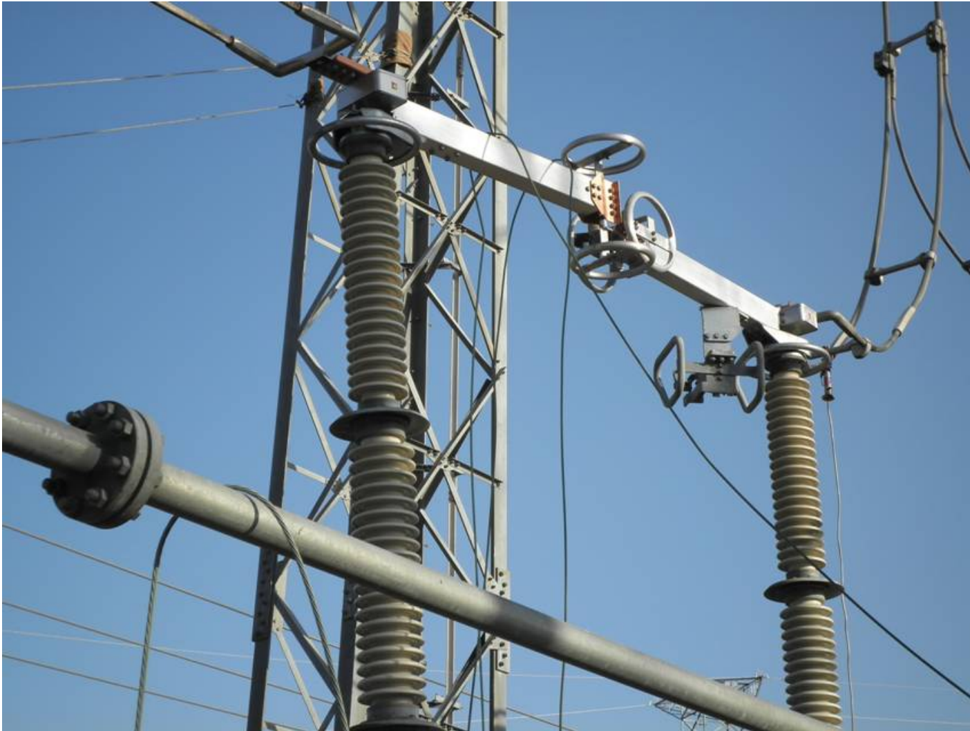
Photo : Tokyo Electric Power Company, March 12, 2011
