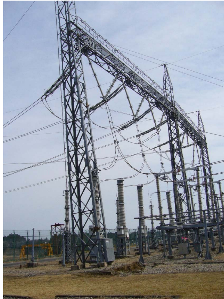
Photo : Tokyo Electric Power Company, March 11, 2011
