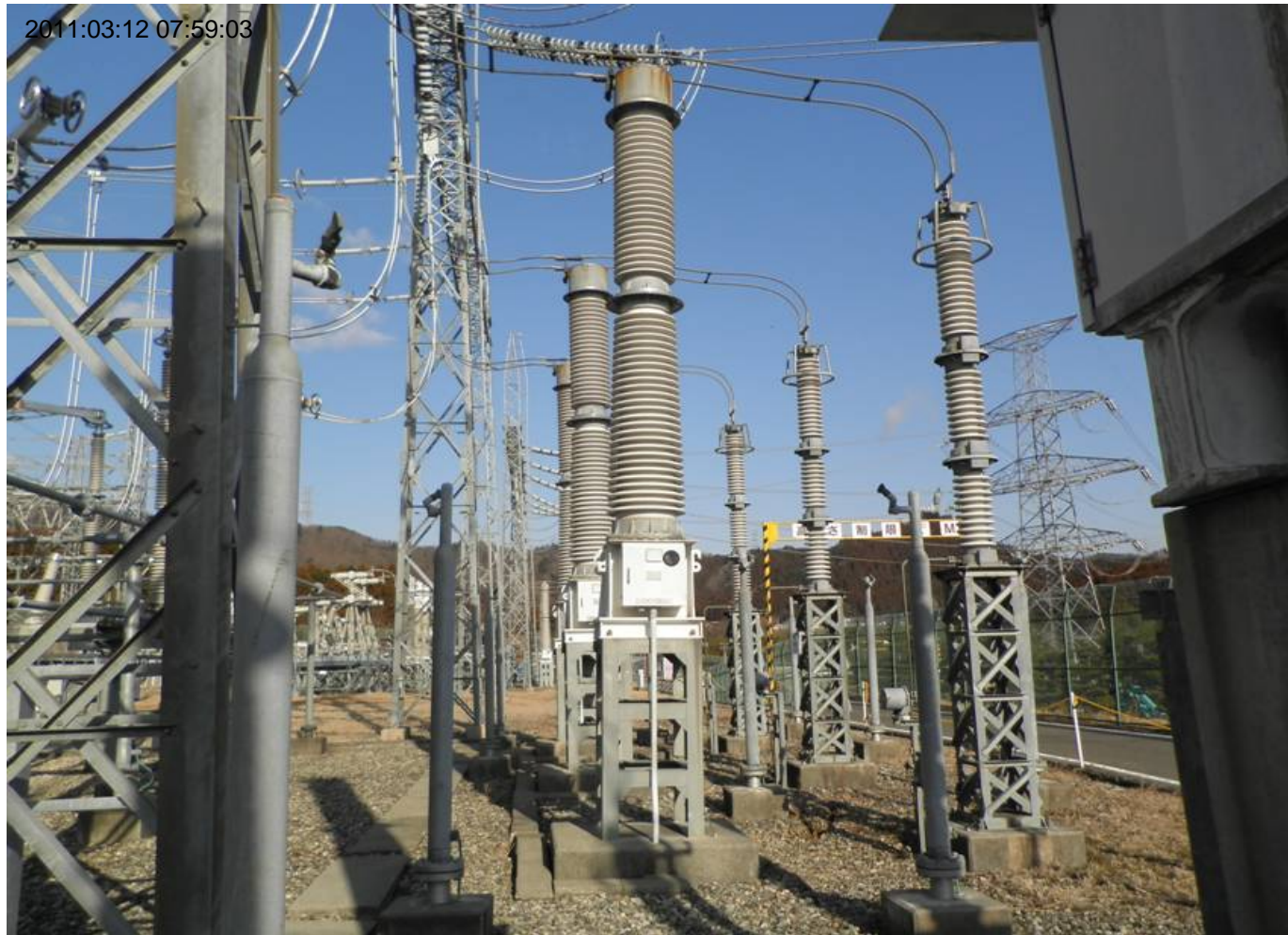
Photo : Tokyo Electric Power Company, March 12, 2011
