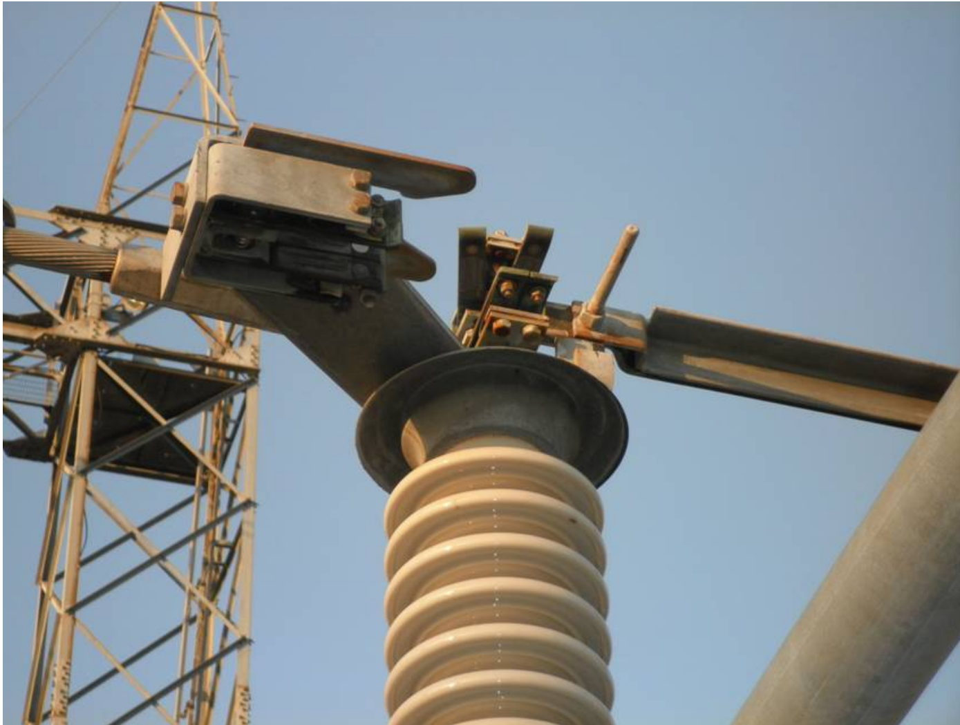
Photo : Tokyo Electric Power Company, March 12, 2011
