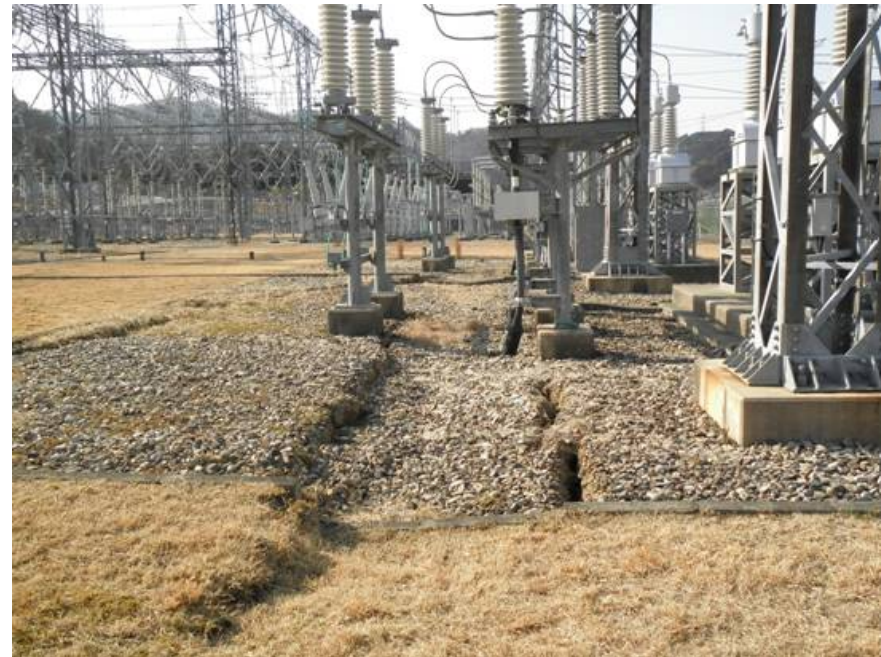
Photo : Tokyo Electric Power Company, March 12, 2011
