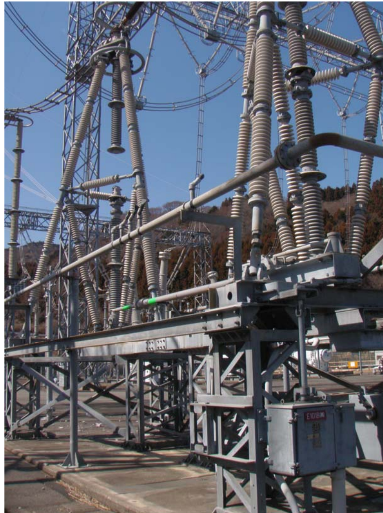
Photo : Tokyo Electric Power Company, March 12, 2011
