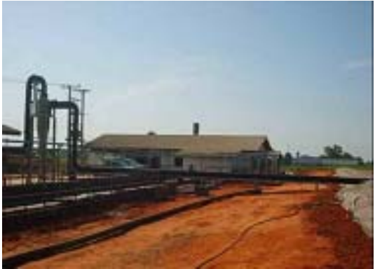
(For reference) Methane recovery facilities
