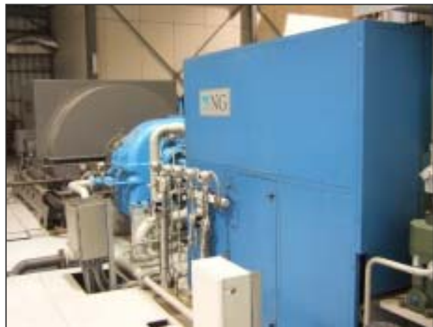
【 Additionally installed generators 】
