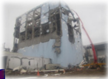
Unit 4 at the accident
