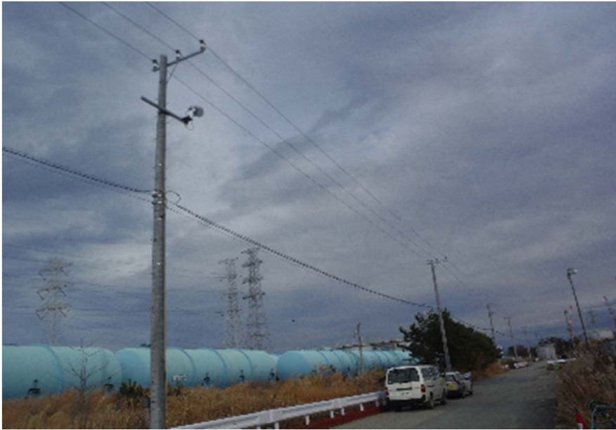
Zone D installation status of distribution lines and lighting facilities
