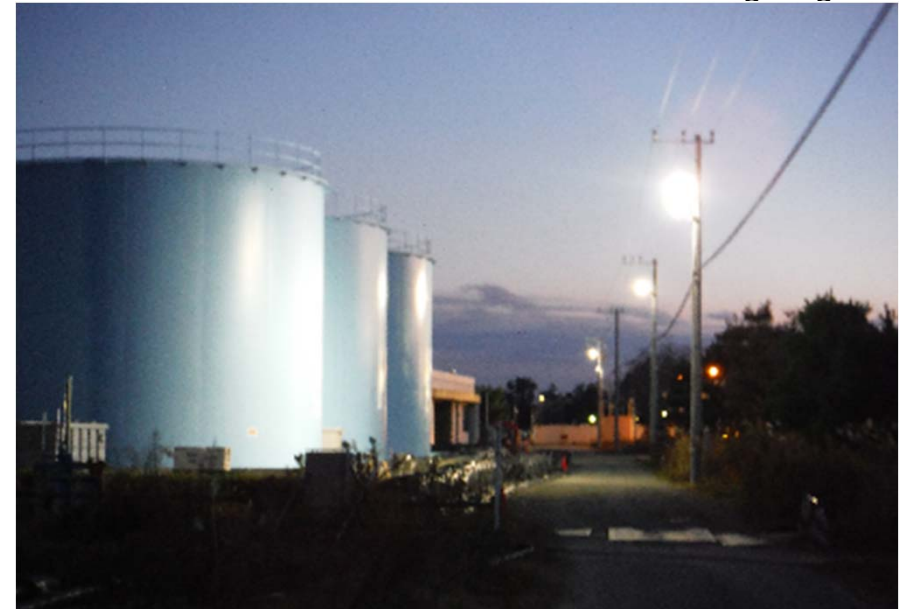
Zone E status of area lighting
