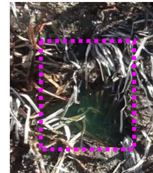
Before debris removal (November 12, 2011)
