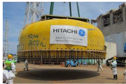
Lifting up PCV upper lid in the upper part of the operation floor
