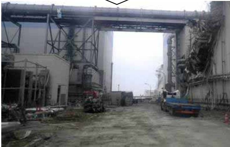
Between Unit 2 and 3
