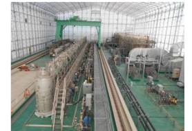
High-performance (multi-nuclide removal equipment)
