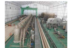
High-performance (multi-nuclide removal equipment)
