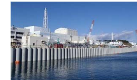
(Sea-side impermeable wall)
