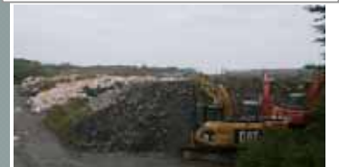
Rubble (outdoor accumulation)
