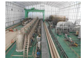
High-performance multi-nuclide removal equipment
