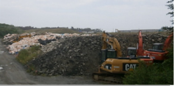
Rubble (outdoor accumulation)
