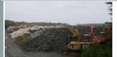
Rubble (outdoor accumulation)
