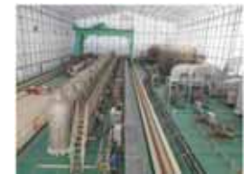
(High-performance multi-nuclide removal equipment)
