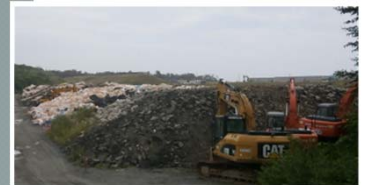
Rubble (outdoor accumulation)
