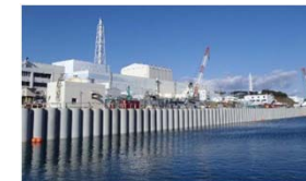
(Sea-side impermeable wall)
