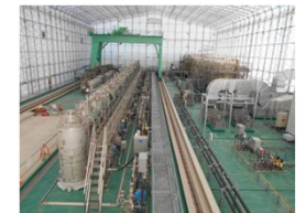
(High-performance multi-nuclide removal equipment)
