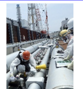
(Opening/closure of frozen pipes)
