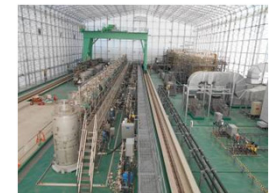
(High-performance multi-nuclide removal equipment)
