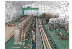
(High-performance multi-nuclide removal equipment)
