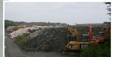
Rubble (outdoor accumulation)
