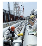
(Opening/closure of frozen pipes)
