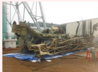
Fuel handling machine removed from the pool
