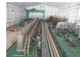
(High-performance multi-nuclide removal equipment)
