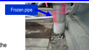
(Land-side impermeable walls; example of freezing functioning test point)
