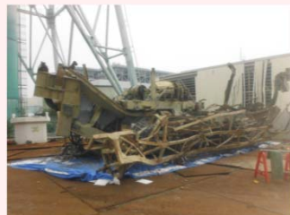
Fuel handling machine removed from the pool
