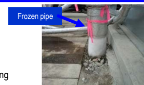
(Land-side impermeable walls; example of freezing functioning test point)
