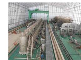
(High-performance multi-nuclide removal equipment)
