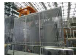
(Installation status of the facility to absorb radioactive materials)
