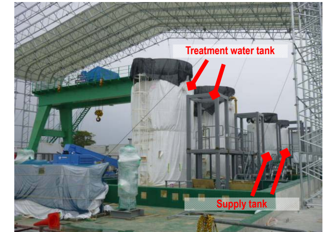
Figure 4: Installation status of high-performance multi-nuclide removal equipment
