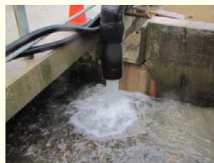
<Water release through the groundwater bypass>
