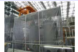
(Installation status of the facility that absorbs radioactive materials)
