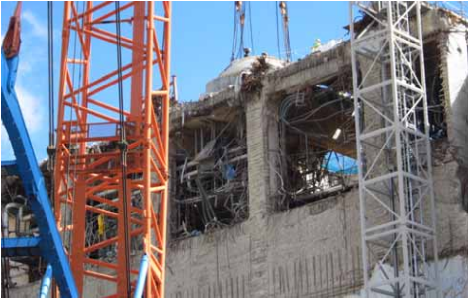
RPV upper lid on the upper part of the operation floor
