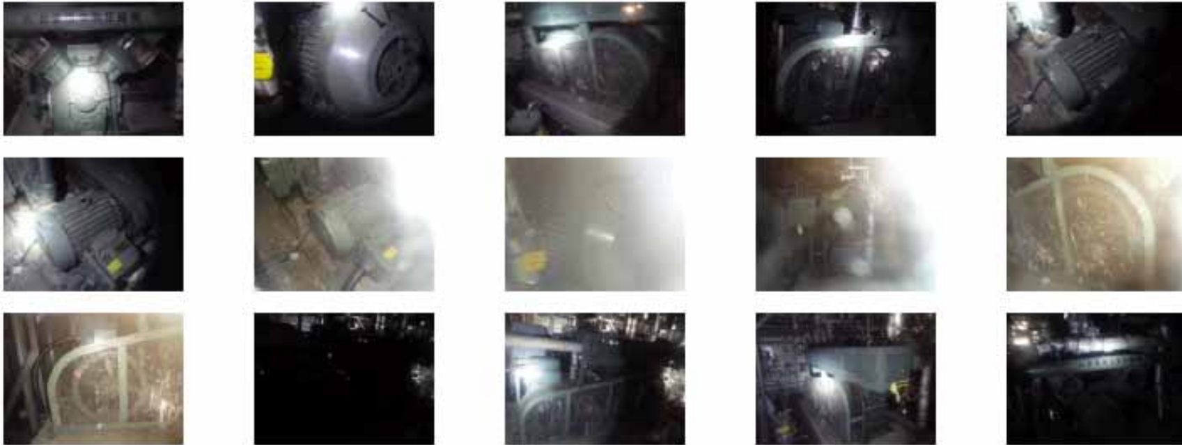
(35)Unit 4 Instrument Air Compressor [Date the photos were taken (gathered): March 25, 2011] Photos taken by a TEPCO employee 15/600 photos
