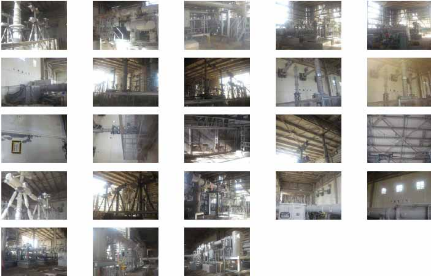
(32)Unit 3 and 4 Ultraigh Voltage Switchyard Area (Inside) [Date the photos were taken (gathered): March 23, 2011] Photos taken by a TEPCO employee 23/600 photos
