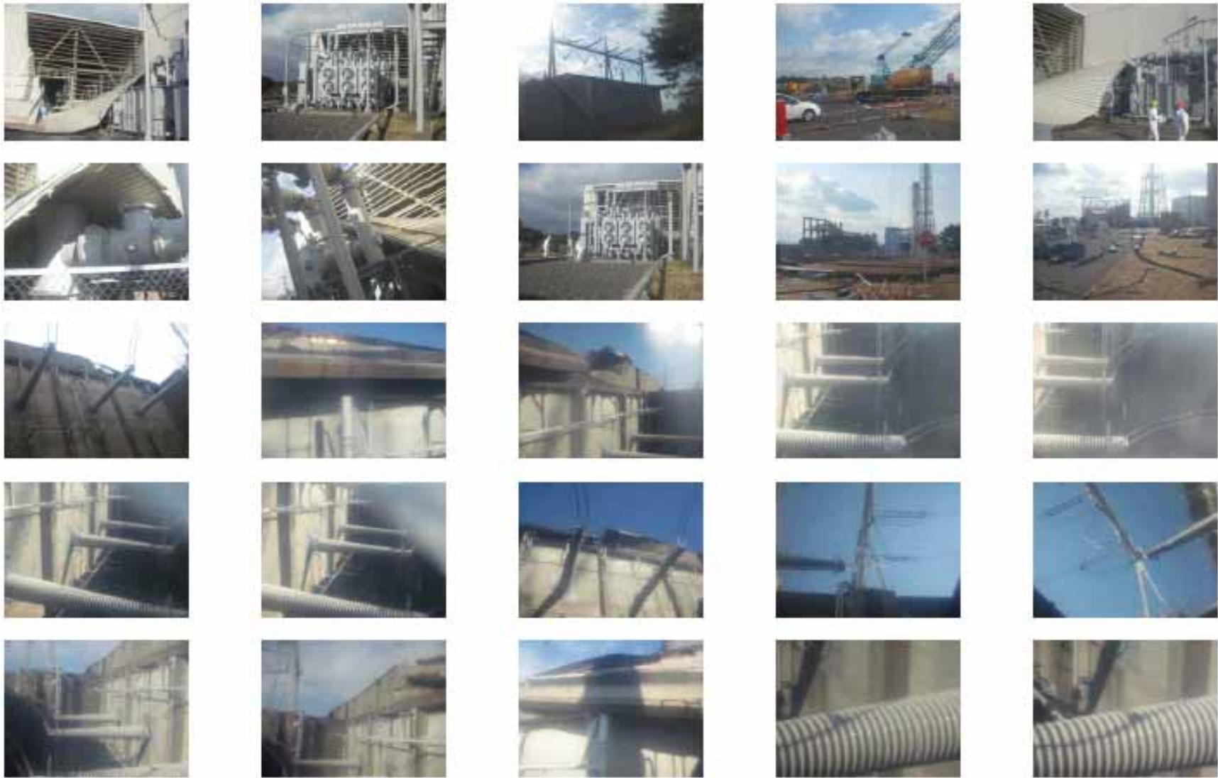
(38)Unit 1 and 2 Ultraigh Voltage Switchyard Area (Outside) [Date the photos were taken (gathered): March 28, 2011] Photos taken by a TEPCO employee 50/600 photos
