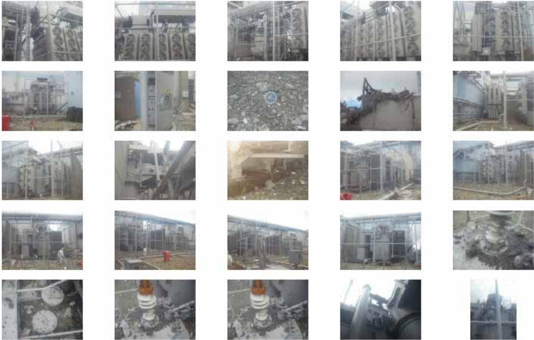
(37)Unit 2 Transformer Area [Date the photos were taken (gathered): March 26, 2011] Photos taken by a TEPCO employee 61/600 photos
