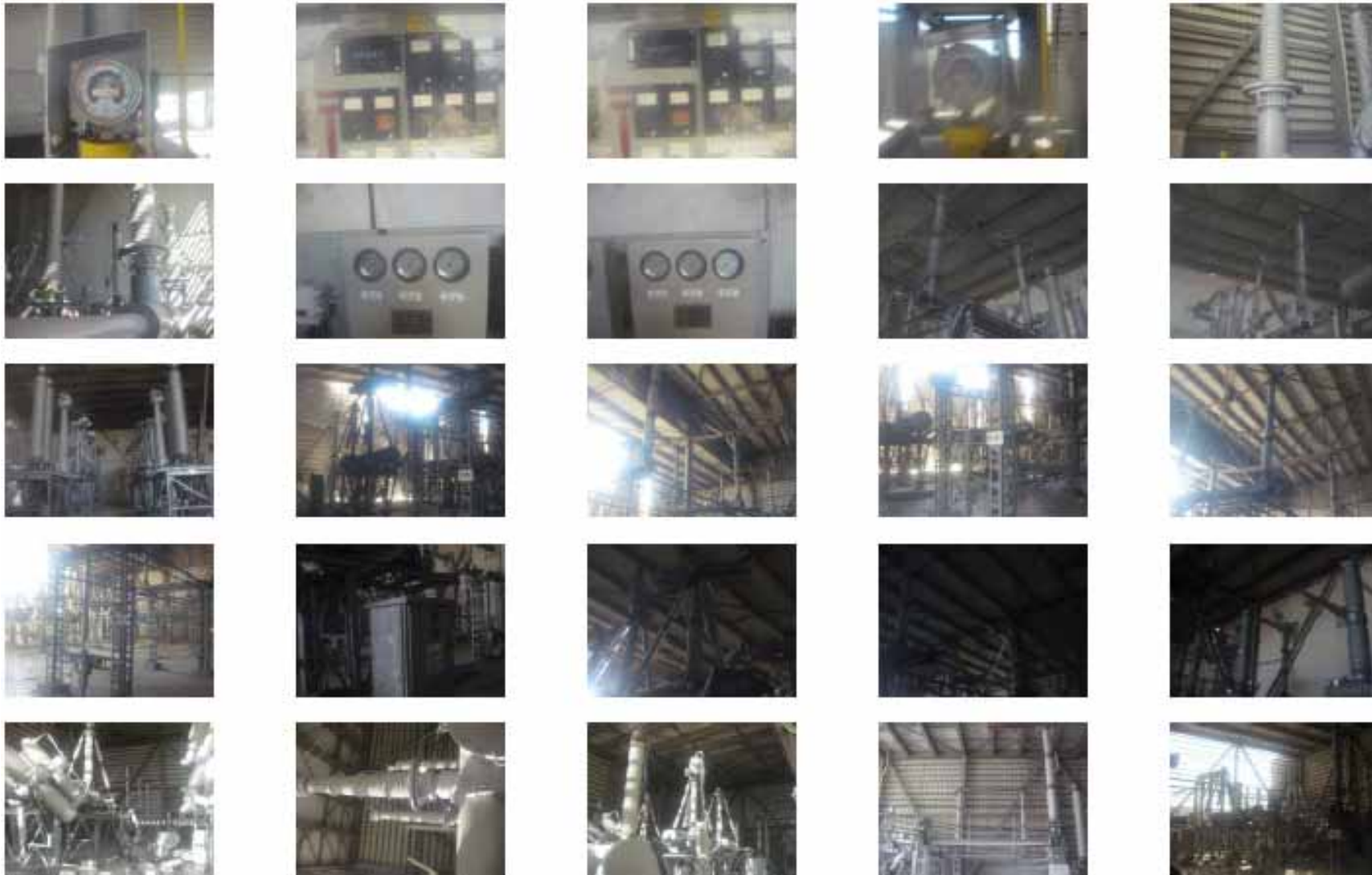
(39)Unit 1 and 2 Ultraigh Voltage Switchyard Area (Inside) [Date the photos were taken (gathered): March 28, 2011] Photos taken by a TEPCO employee 65/600 photos
