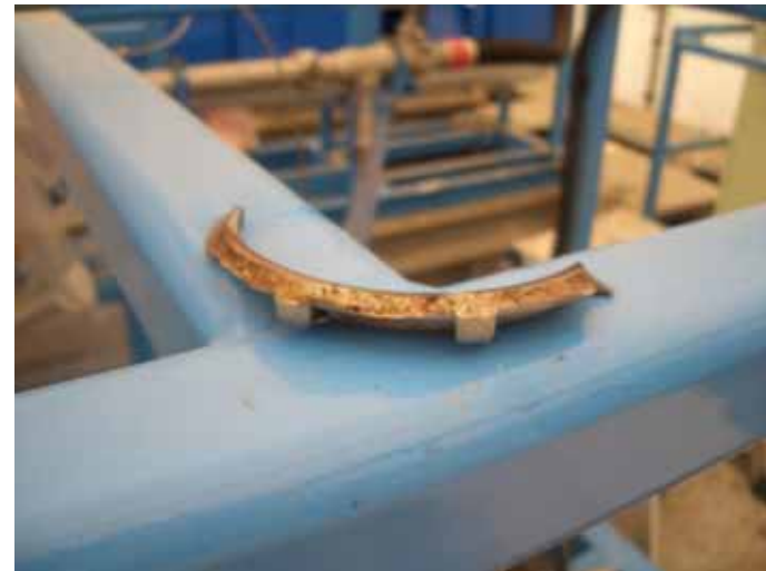
Damaged joint area
