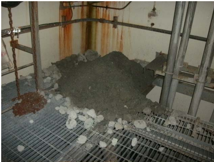
5. Trace of water flowing in (Sand below the penetration area on the ceiling)
