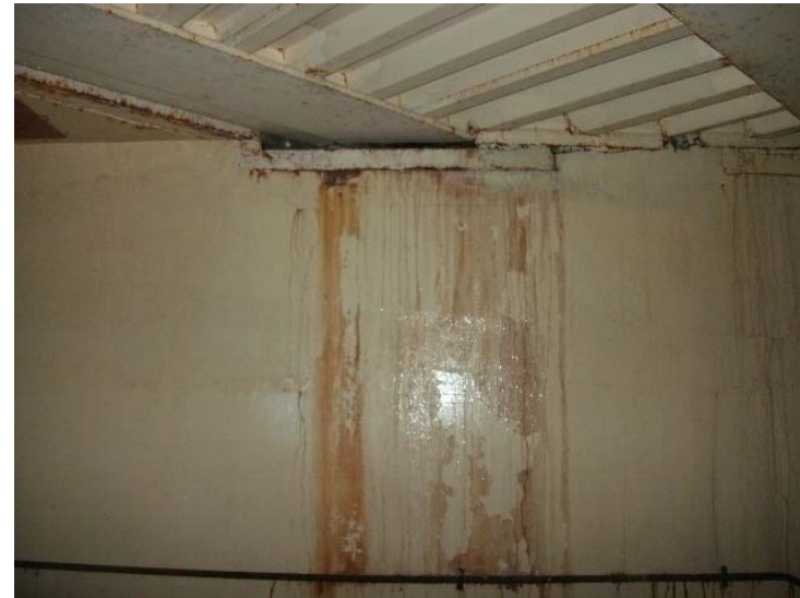
4. Trace of water flowing in (Where the ceiling touches the wall)
