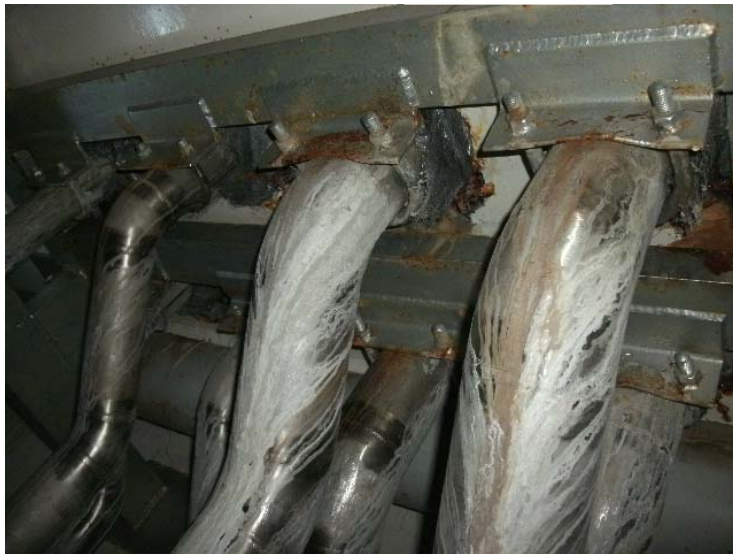
2. Trace of water flowing in (Penetration area on the ceiling)
