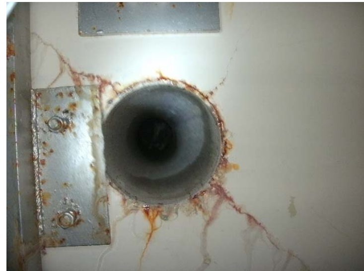
6. Trace of water flowing in (The penetration area on the ceiling above the sand)
