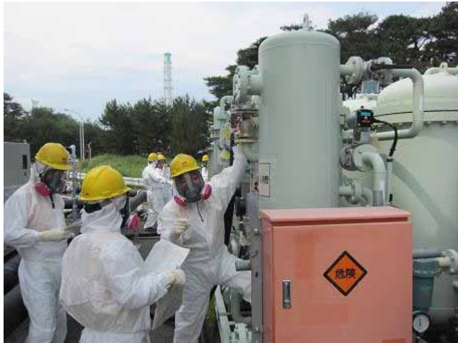
Start-up operation of the emergency nitrogen gas separator (PSA5)
