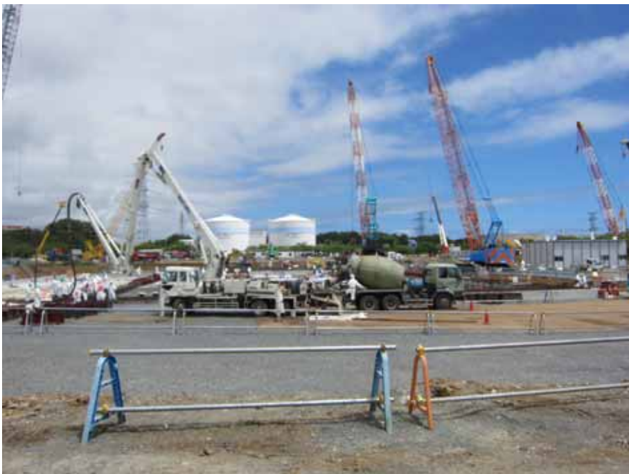
-1 Multi-nuclide Removal Facility construction site (Full-view) Photo taken by a TEPCO employee on June 11, 2012
