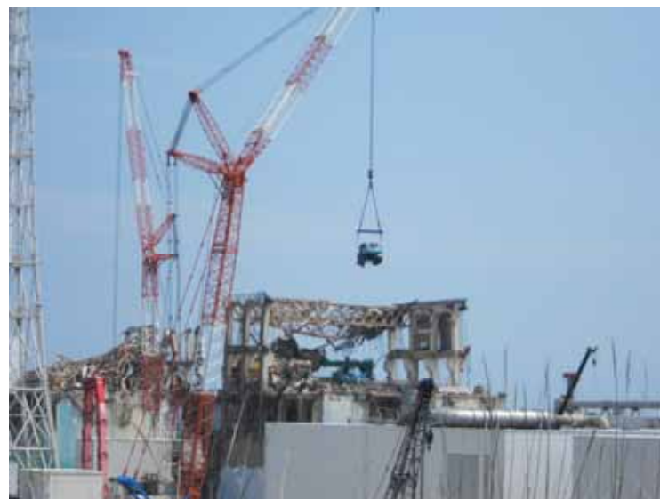
-4 Appearance of Unit 4 (View from the southern hill): Lifting heavy machinery down from the operation floor Photo taken by a TEPCO employee on June 18, 2012
