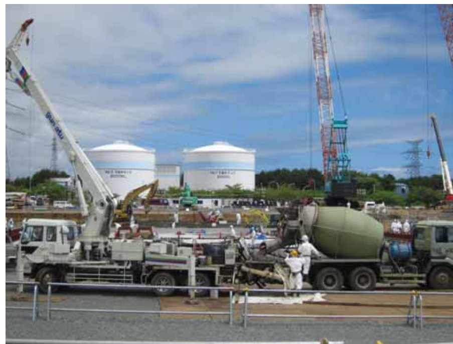
-2 Multi-nuclide Removal Facility construction site (Full-view): Foundation improvement work Photo taken by a TEPCO employee on June 11, 2012
