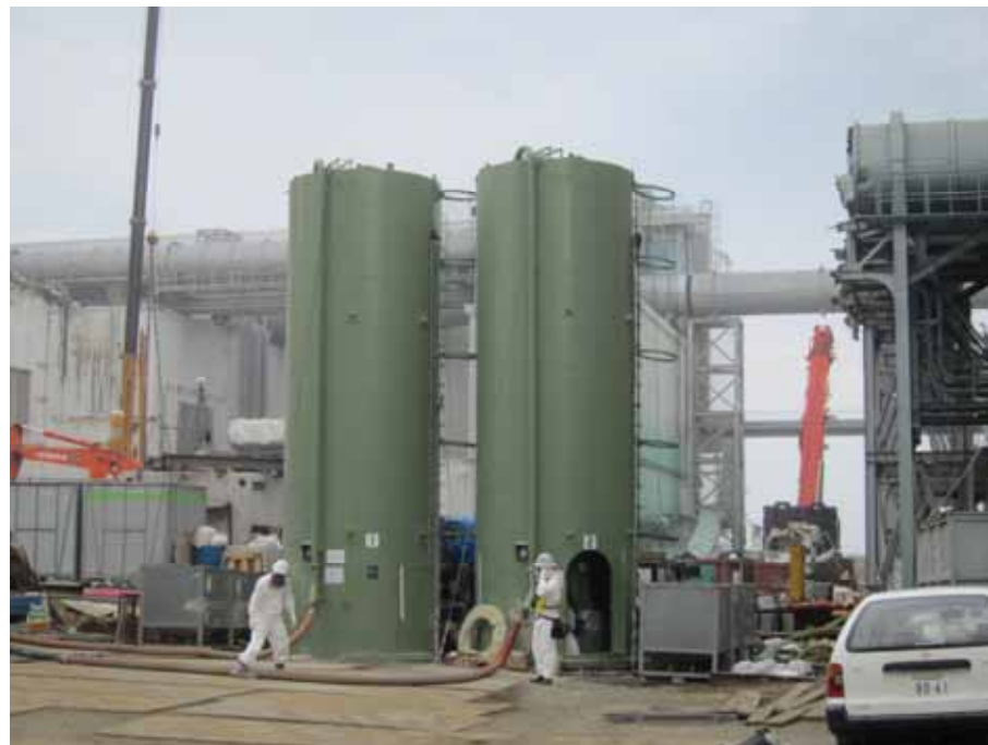
-2 Unit 4 south side foundation improvement work: Cement silo Photo taken by a TEPCO employee on June 7, 2012
